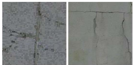
Figure 7 Four examples of cracks in exterior wall
