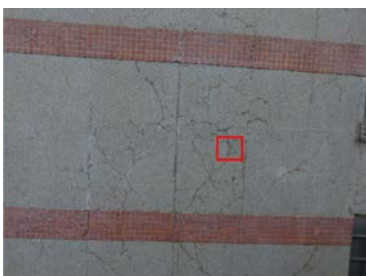
Figure 5 Original image of crack in exterior wall
